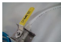
To a valve located at the washout station
